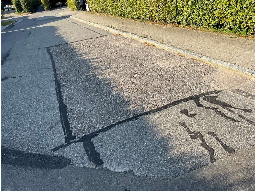
Figur 4.3.4 Manglende retablering af slidlag.
